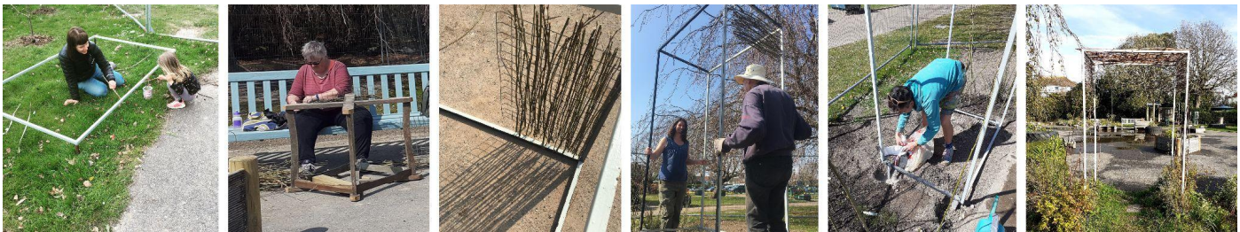
Creating a reclaimed metal 'doorway' with living willow planted to form a natural arch as it grows.
